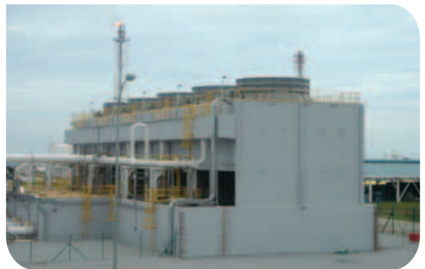
:: Malacca Cogen Power Plant, 12,500 m 3 /hr (5 cells).
