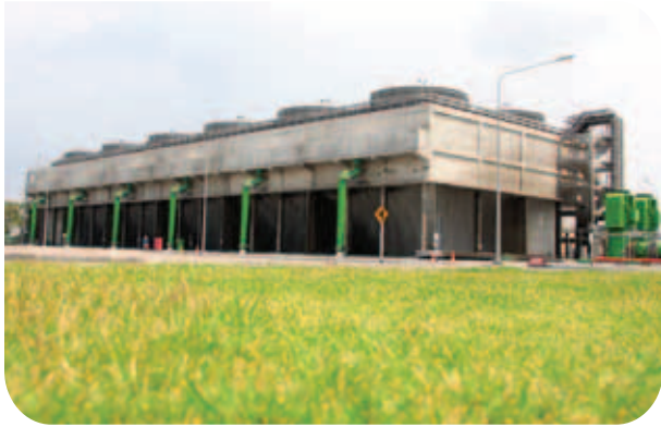
:: Bangpakong Combined Cycle Power Plant, Thailand 35,800 m 3 /hr (12-cell back to back).
